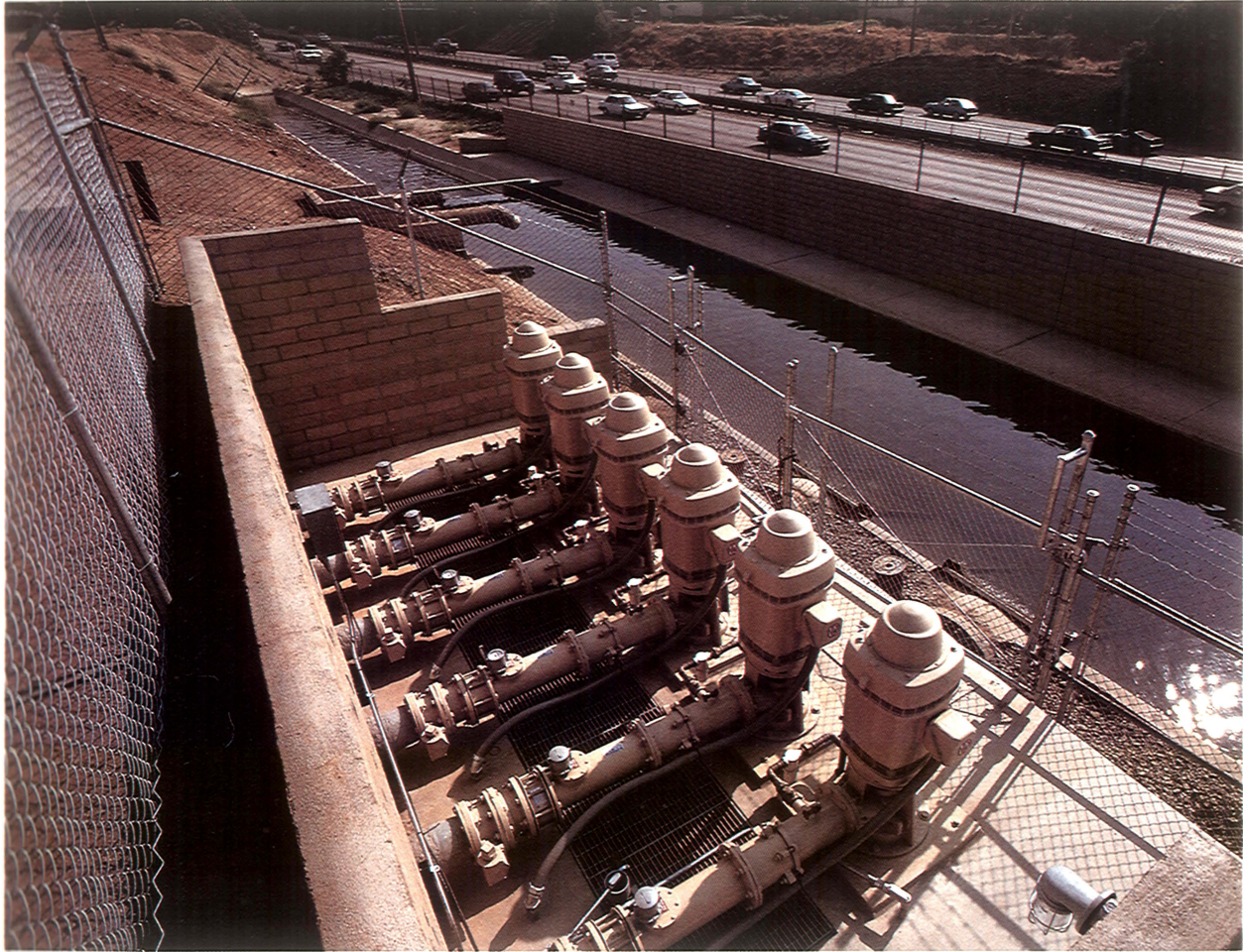
This year, the Water Utility completed construction of a new six-pump booster station at the Olivewood Booster Station, allowing Riverside to exchange agricultural water for potable water from the Gage Canal.
