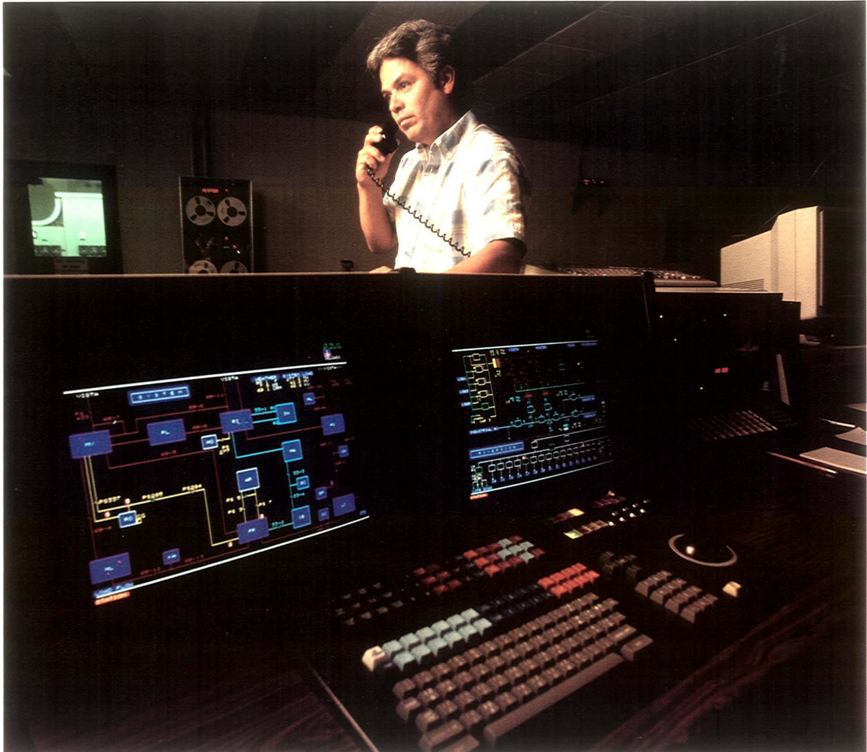
The Electric Utility's system operating, monitoring, and dispatching facility operates the system for regular maintenance and construction as well as working to keep customers in service if there is a problem. Last year the system operated over 99.99% of the time.
